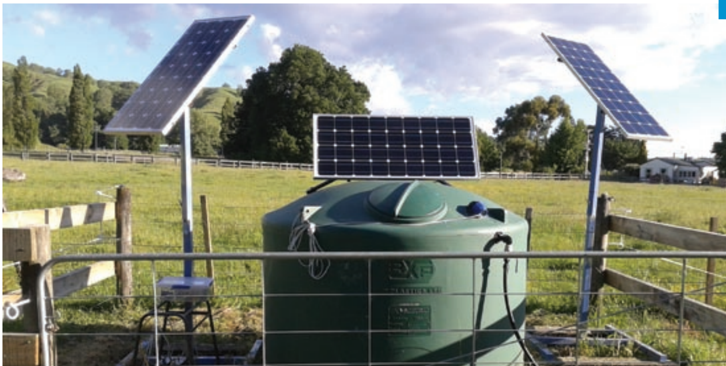
ABOVE: Midsize 240 watt solar pump system
